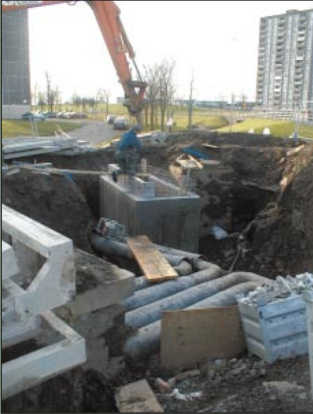
Civil engineering and services contracts are complex and will cause some traffic disruption.
