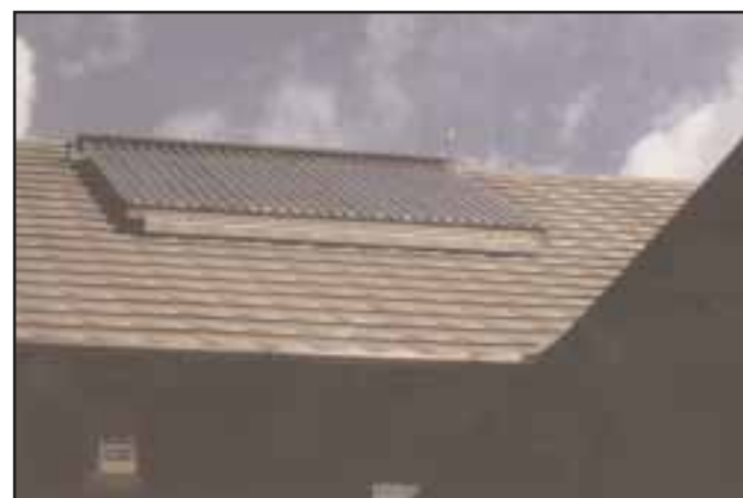
SOLAR PANEL IN ROOF
